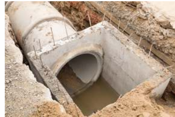
Storm Sewer Line
